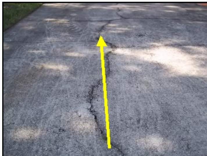
Need to be repair
